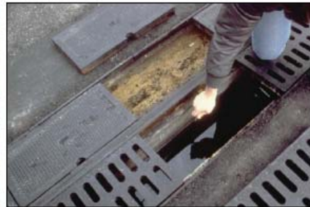
Perimeter Sand Filter
