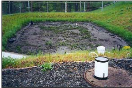
Surface Sand Filter
